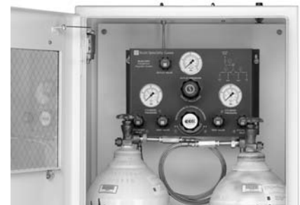
Gas Cabinet with Model 8404 ChangeOver
